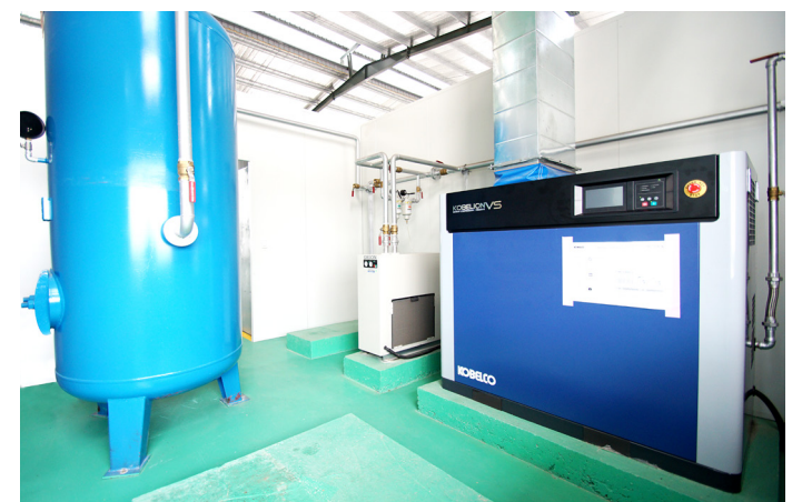
Compressor and Air filters system
